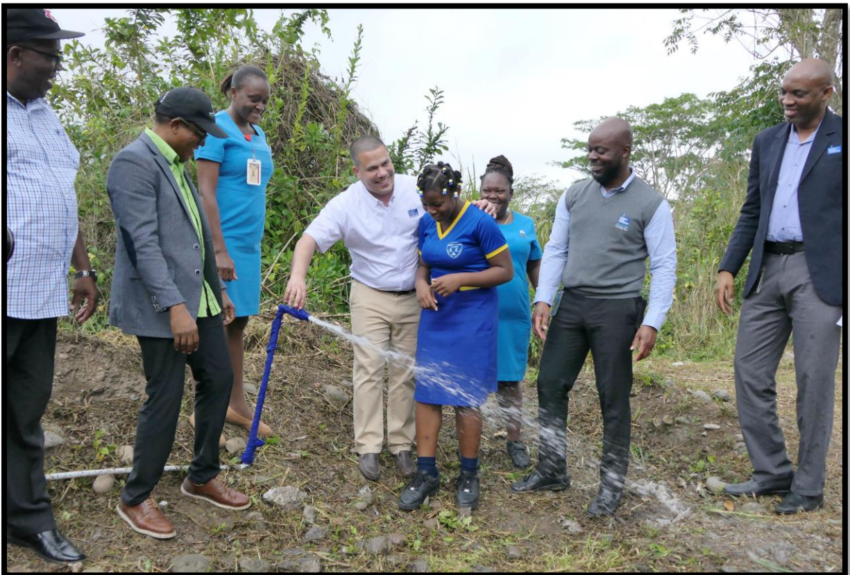
Senator Matthew Samuda (centre), Minister without Portfolio in the Ministry of Economic Growth and Job Creation, shares a laugh with Bromley Primary student Hadasia Thompson while turning on the pipe during the commissioning ceremony for the Macka Hill Pipeline Replacement Project in St Mary. Joining in the activity are (from left) Councillor for the Belfield Division, Levan Freeman; Dr Norman Dunn, the Member of Parliament for St Mary South Eastern; community health aids Alicia Wilson and Evette McLaughlin; Acting Vice President of Operations at NWC, Herman Fagan; and Acting Regional Manager for St Ann, St Mary and Portland, David Pryce.
